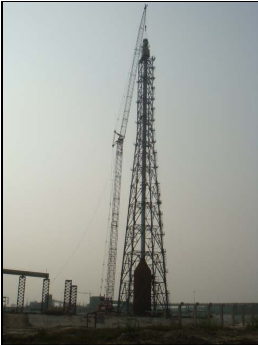
Erection (In-progress) of 72" dia. x 119m NCU HC Flare at IOCL Panipat Refinery, Panipat Naphtha Cracker Project (EPCC-9)
