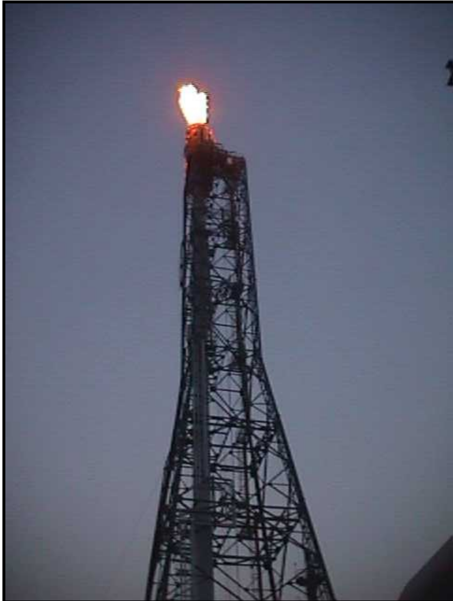
Flare (72" dia. x 100m high) in operation at IOCL Barauni Refinery
