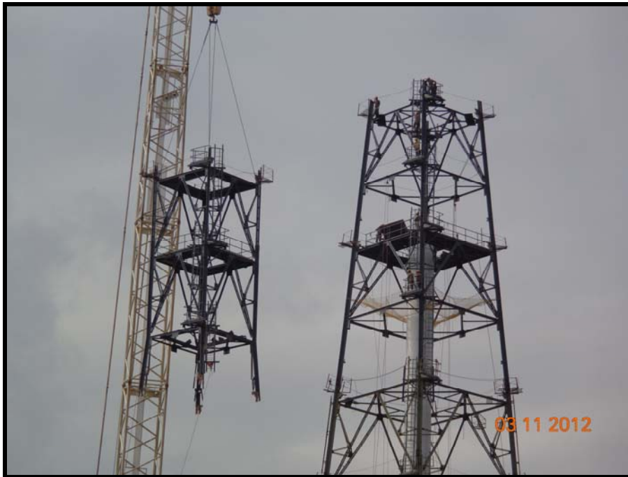
OMPL: Erection in progress of Derrick Structure (122.5 m high) and Flare Stack Riser (72" NB dia.)
